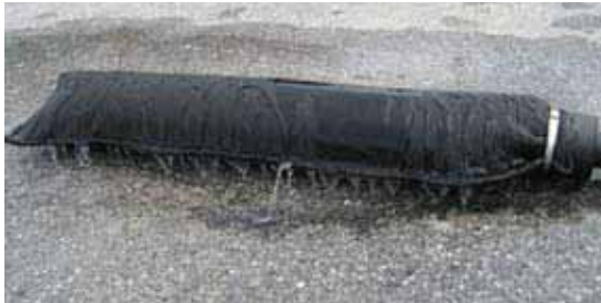
EVAC Filtration System filtering water.
